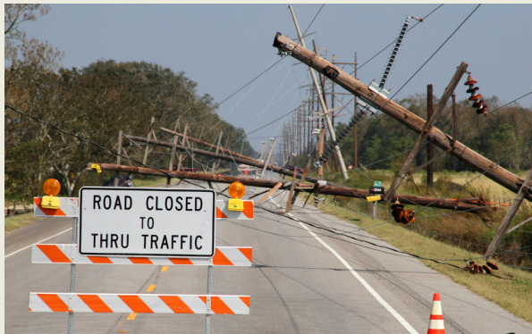
DOWNED ELECTRIC LINES - ELECTRICAL CO-OPS
