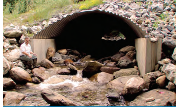
Infrastructure Project and Natural Systems Protection: This reconstructed culvert in Moosalamoo National Recreation Area in Arlington, Vermont uses rocks and sand to simulate a natural fish passage.
