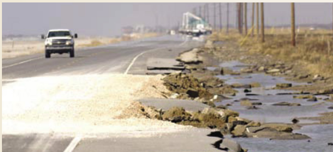
BEFORE MITIGATION: ROAD NEAR HOLLY BEACH ERODED
