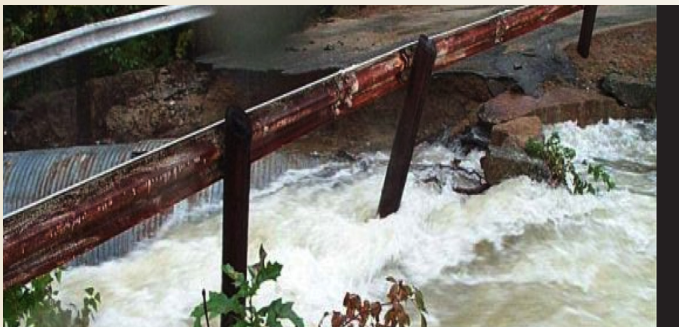
BEFORE MITIGATION: CULVERTS WASHED OUT DURING EVENT
