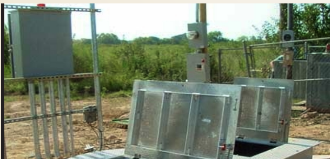
AFTER MITIGATION: PUMP STATIONS WITH ELEVATED CONTROL BOX
