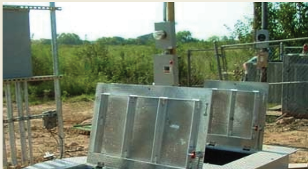
AFTER MITIGATION: PUMP STATIONS WITH ELEVATED CONTROL BOX
