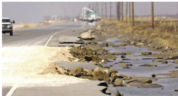
BEFORE MITIGATION: ROAD NEAR HOLLY BEACH ERODED
