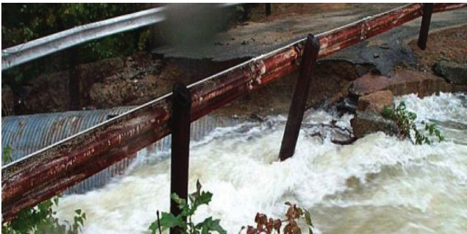
BEFORE MITIGATION: CULVERTS WASHED OUT DURING EVENT
