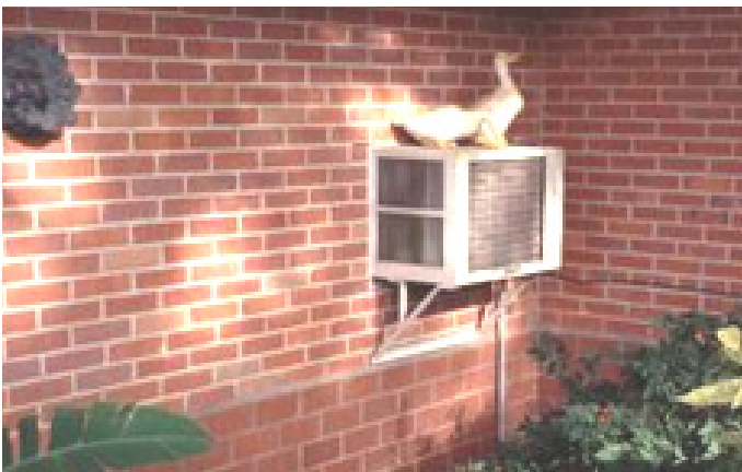
Figure 17 - This Baton Rouge, LA home had thin facing brick placed over the waterproofing materials.
