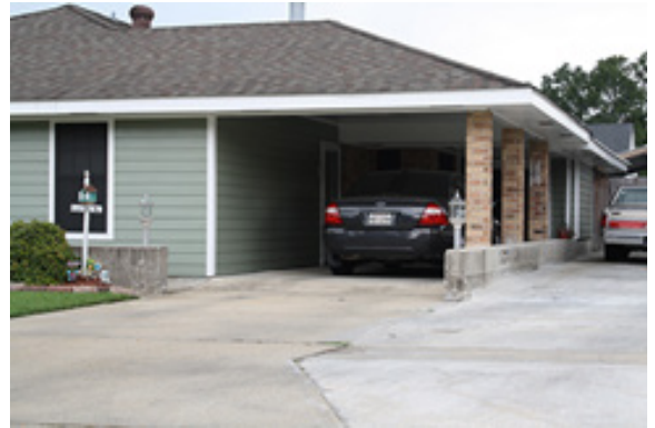
Figure 15 - This home is surrounded by a floodwall that doubles as a planter. The driveway must be sandbagged during a flood event.
