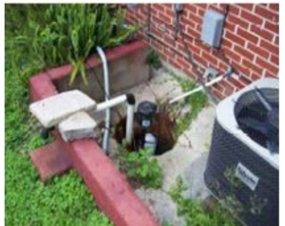
Figure 14 - A small flood wall stops the water from entering the house. If water overtops the wall, it collects in this basin, or sump, and is pumped out by a sump pump.
