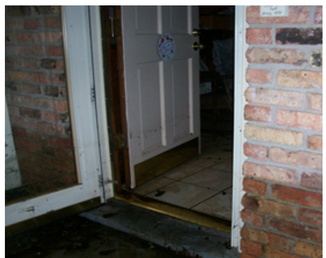
Figure 16 - Flooding of this slab-on-grade house was up to 11/2 feet. Damage could have been prevented by dry floodproofing.
